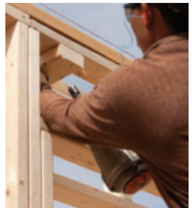
Nail penetration through the lumber is a special concern where the piece is held in place by hand
